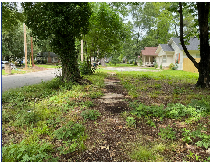
Looking N along damaged sidewalk path at property frontage
